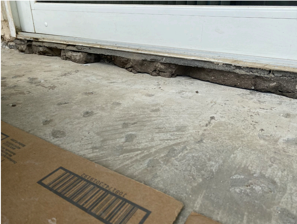
Picture 1: Cracked topping at Unit 207
