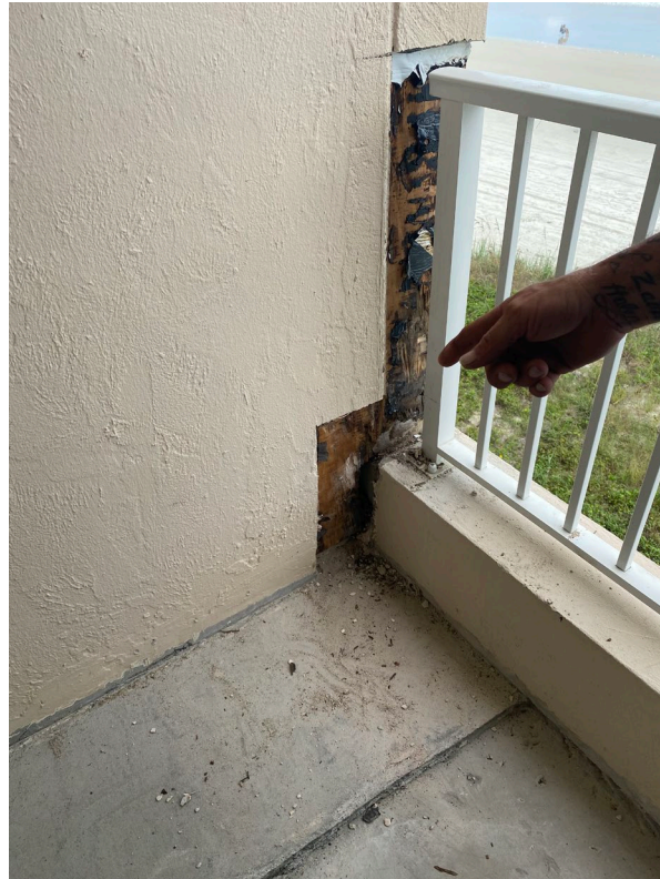
Picture 2: Typical rotten plywood sheathing
